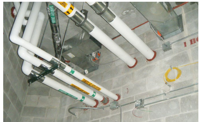
Fire stopping of services using proprietary fire sleeving.
